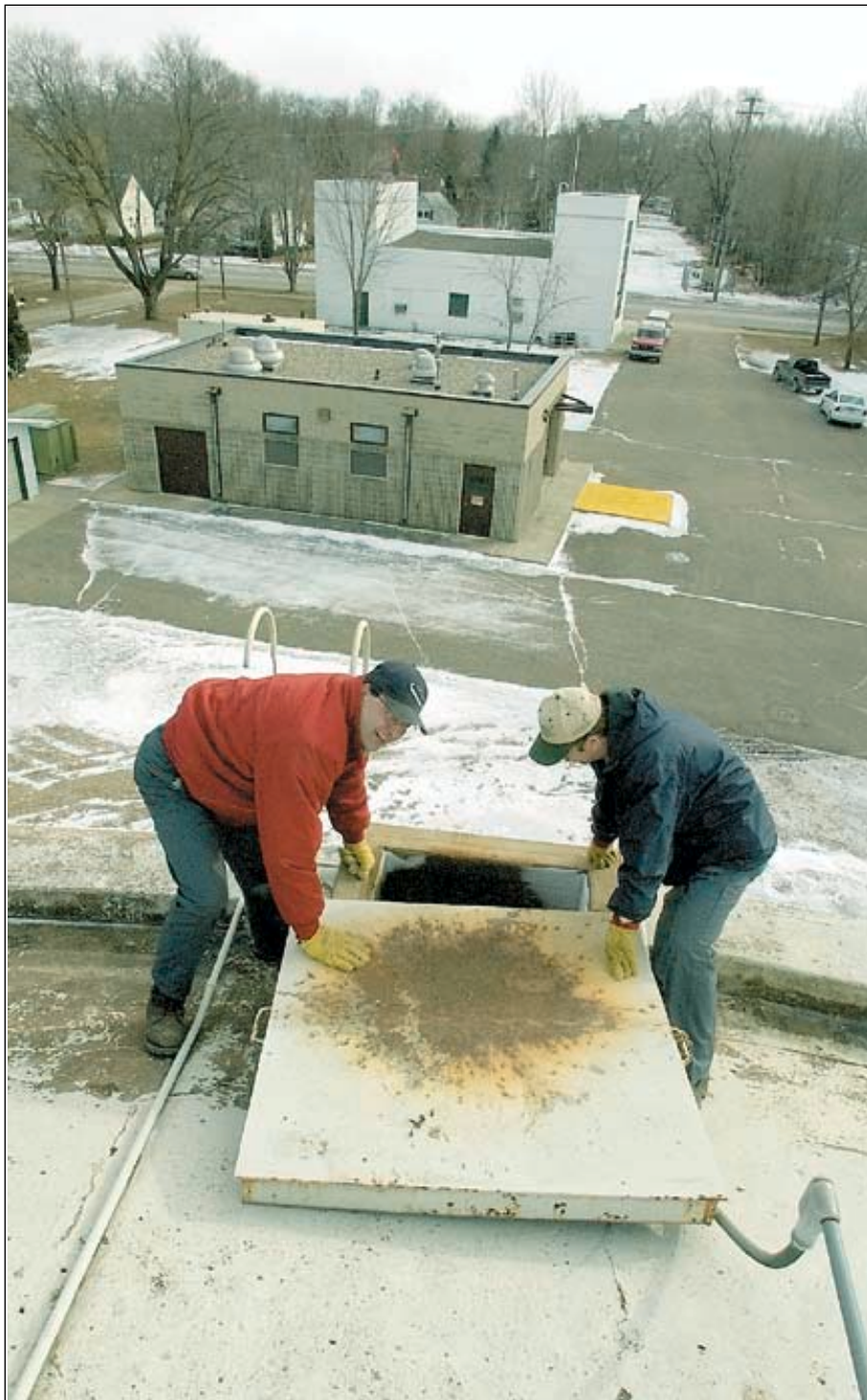
Dennis Duchene, superintendent of Faribault's water department, left, and foreman Jim Hausen look inside the water reservoir at the Faribault Water Works Station on Monday. Behind them are the chemical feed building and the pumping station. (Kelli Wencil / Daily News)
